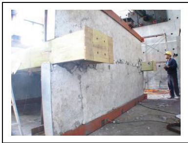
Figure 6. Crack at the top slab
