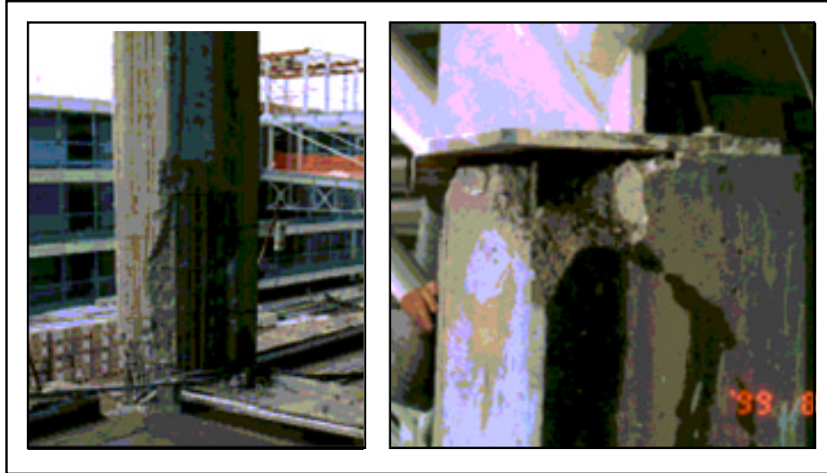
■ Figure 3. Observed Damage to the Terminal Building; base of third story column (left) and base of roof truss connection to column (right)
