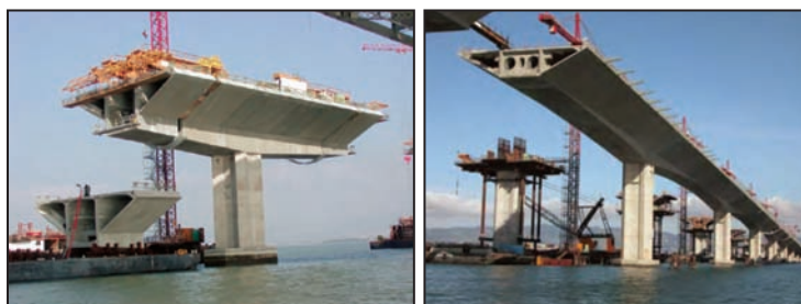
Use of prefabricated segmental construction is one way to accelerate bridge construction. Here, hinge pipe beams at mid-span expansion joints are being incorporated in the San Francisco - Oakland Bay Bridge
