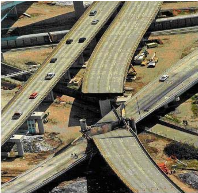
Figure 2: View of damage from above
