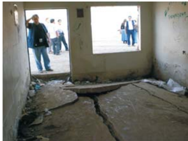
House settlement and floor cracks
