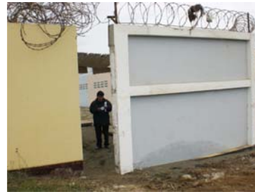
Lateral spread. The right wall has moved to the right and towards the reader, “opening a door”.
