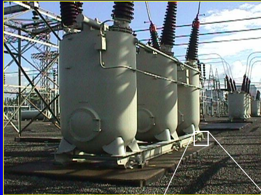
Bulk Oil Circuit Breaker
